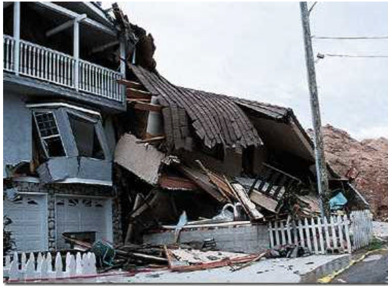
Aftermath of the 1995 La Conchita landslide, in southern California. (Photograph by Robert L. Schuster, USGS.)
