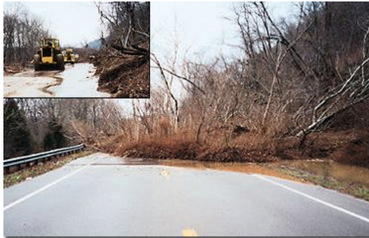
March, 1997: landslide damage on portions of U.S. Route 52, along the Ohio River Valley, after eight inches of rain fell in just two days. (Photographs by Aaron Mitten, Ohio Department of Transportation.)
